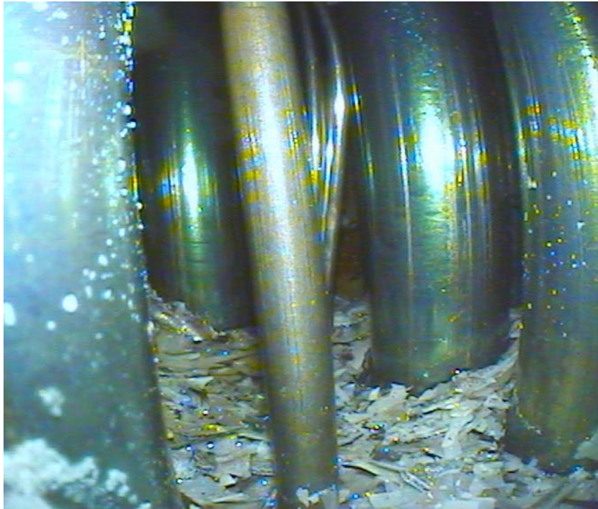
debris at the bundle bottom
