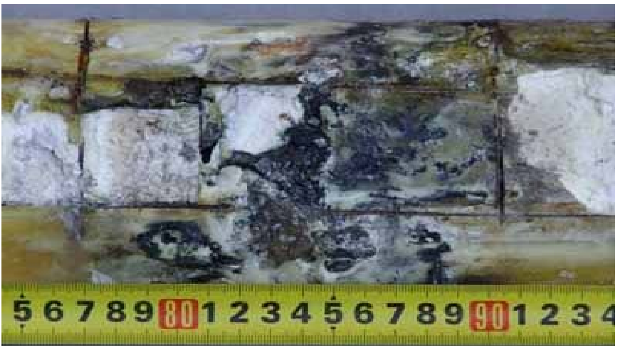
Fig. 4. External appearance of the thermoinsulation with traces of melting at the level of 700 – 1000 mm.
