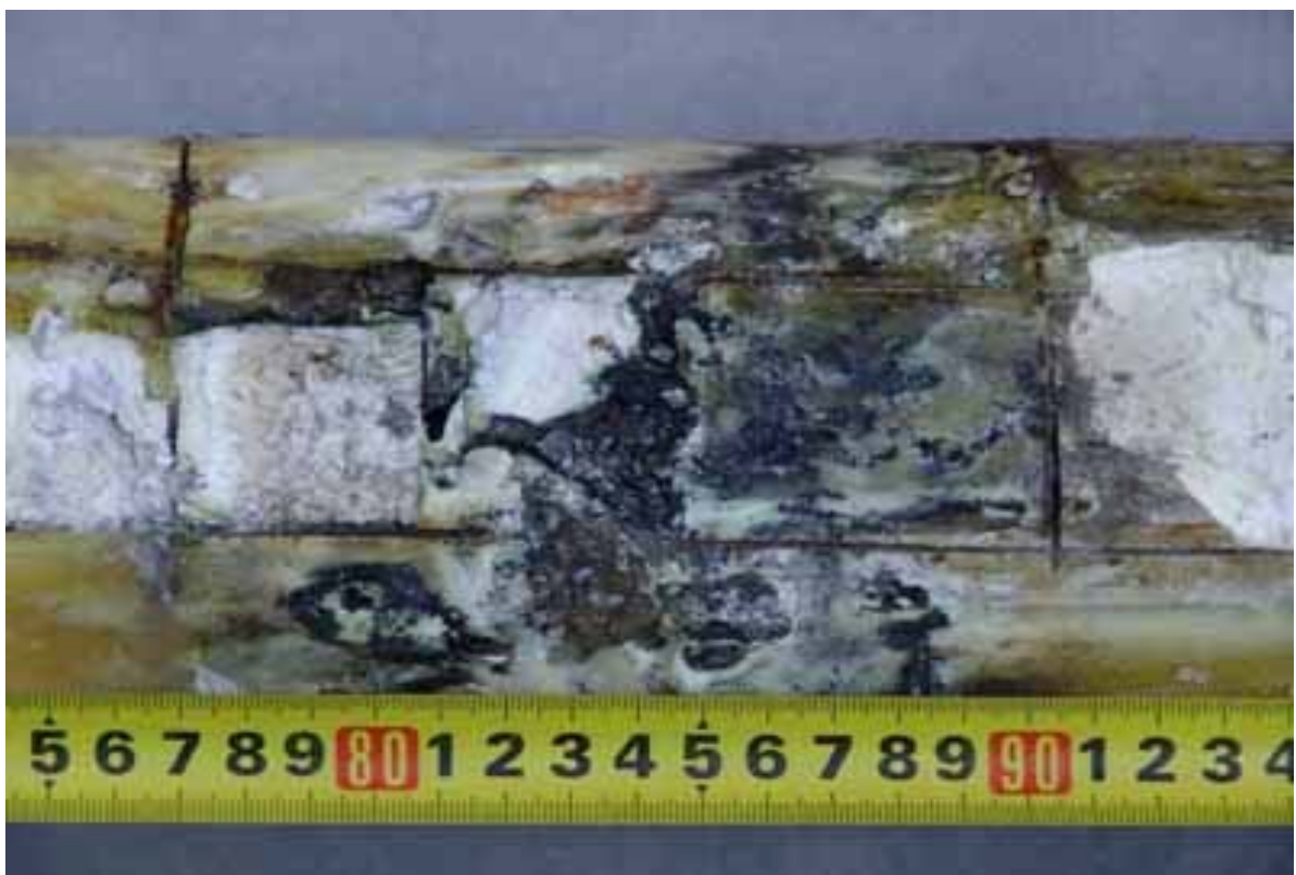
Fig. 23. View of thermoinsulation with traces of melting at the level of 700 – 1000 mm.
