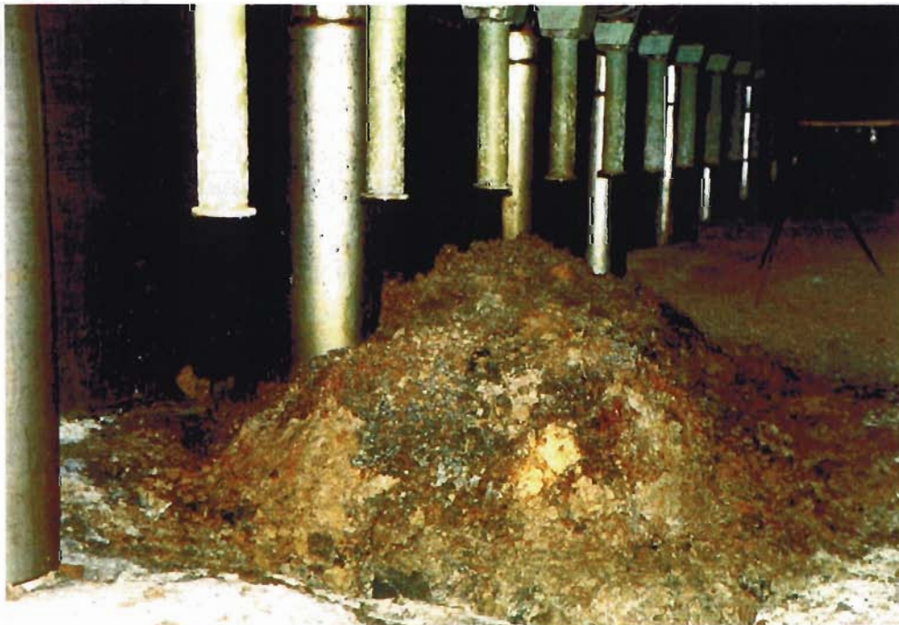
Fig. 5.15. LFCM "pile" on the first floor of pressure- suppression pool, Room #012/7
