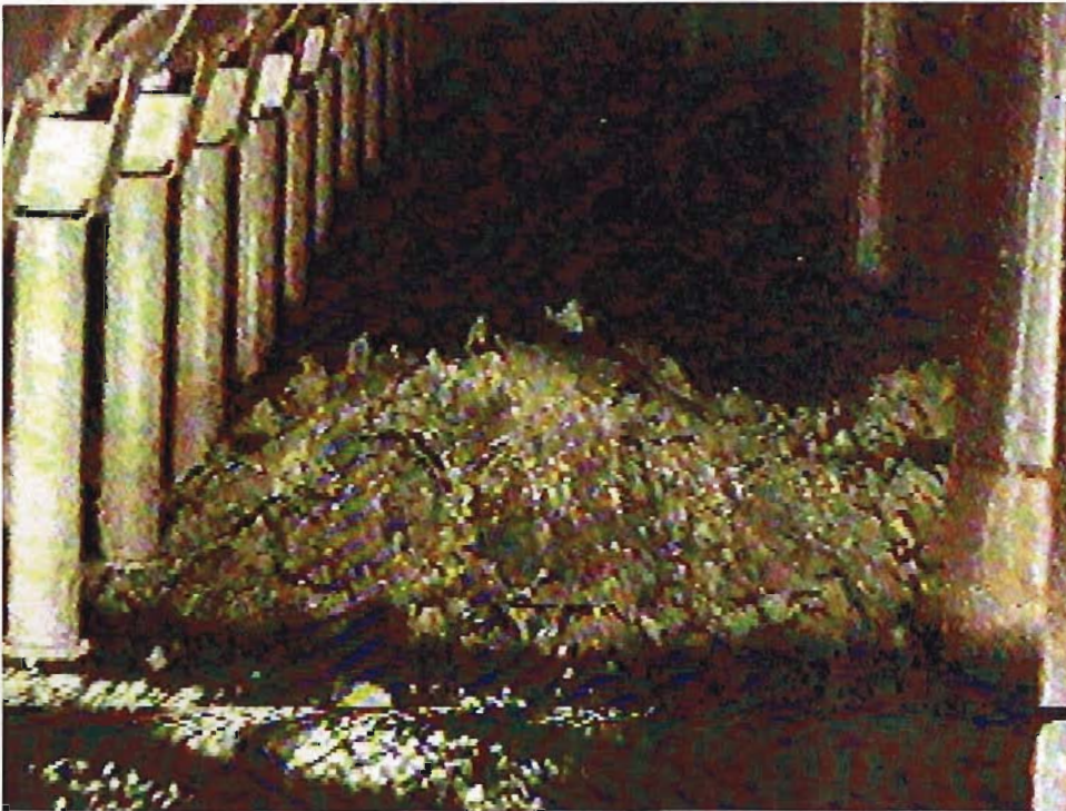
Fig.5.14. LFCM "pile" on the second floor of pressure- suppression pool, Room 012/15
