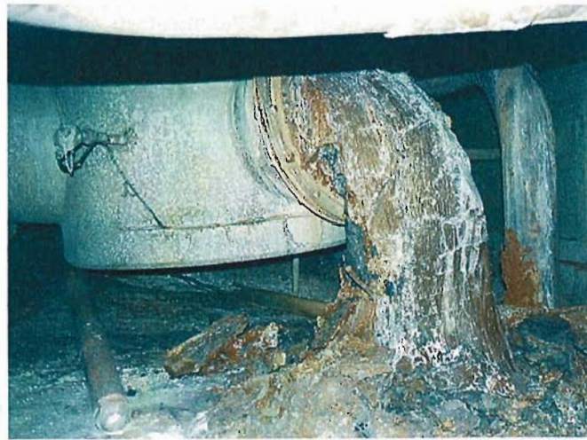
Fig.5.17. Solidified “jets” of LFCM flowing out of the 4th steam-distributing valve to Room #210/7
