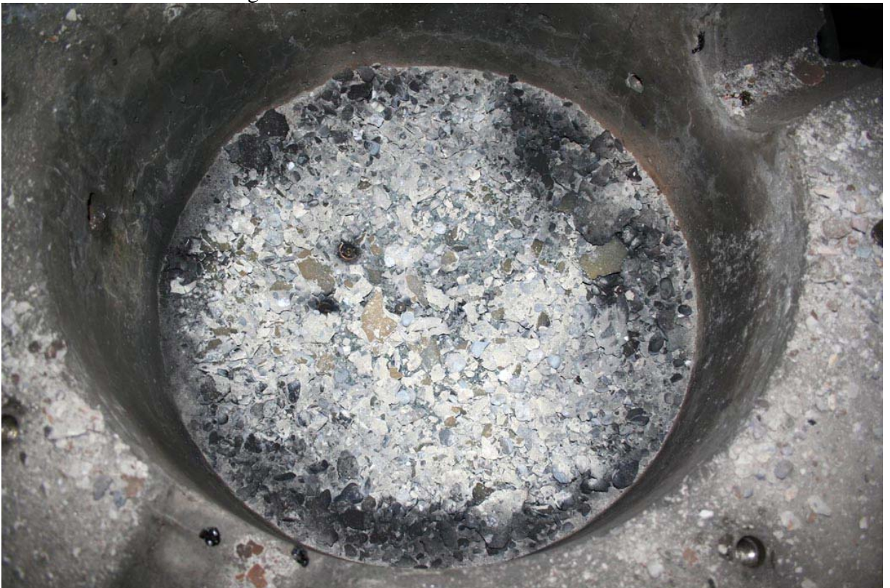
Fig. 8 – Degraded surface of concrete base under RPV model
